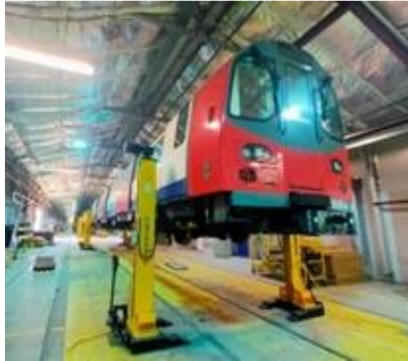
Figure 3: New Jacks installed in the TFOS
