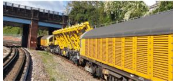
Figure 10: Kirow wagon hauled by battery locomotives
