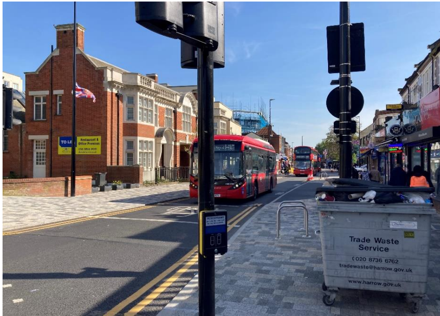
Figure 4 - Construction recently completed on major bus infrastructure in Wealdstone Town Centre (Harrow), including new footways, cycle parking and greening
