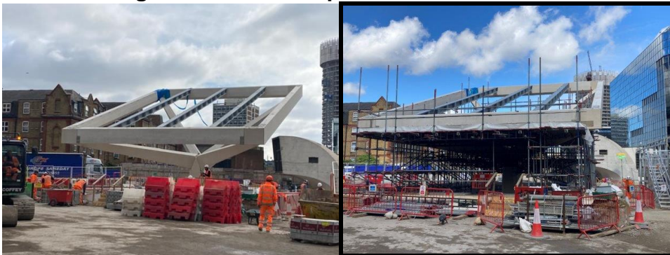
Image 1 - Main Station Entrance Installation of 4 precast concrete tree arms and steel ring beam – March/April 2022
